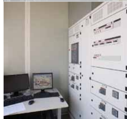
➤ control and supervision room
