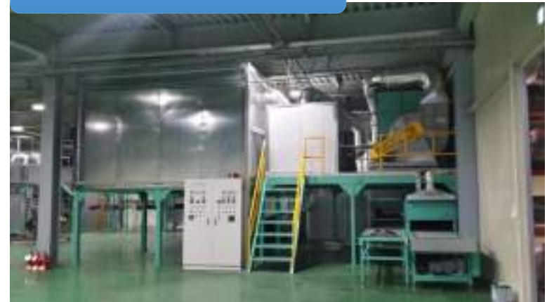
BELT CONVEYOR Line
