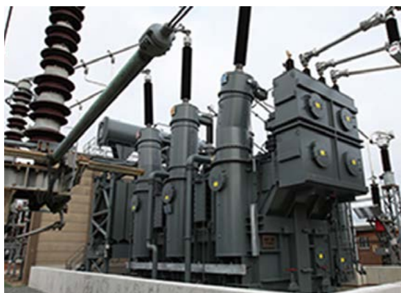
Power Transformer for Substation
