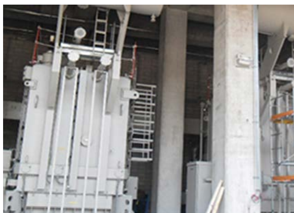
Power Transformer for general Factory
