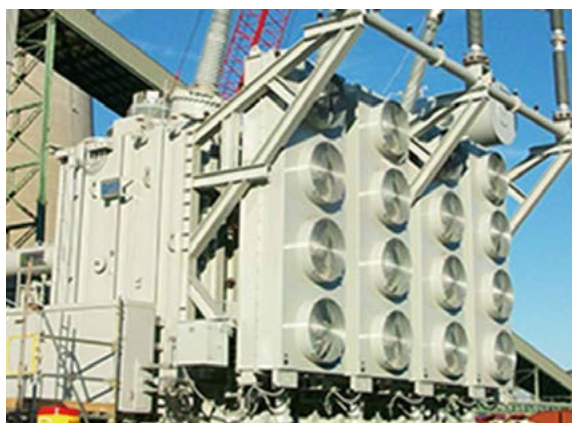
Power Transformer for Power Plant
