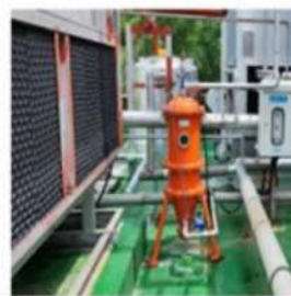
[Namyang Dairy's Gyeongju Plant]
