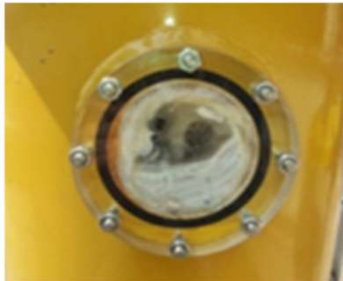
The scale collection shown in the inspection window
