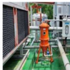
[Namyang Dairy's Gyeongju Plant]
