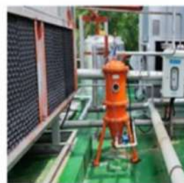
[Namyang Dairy's Gyeongju Plant]
