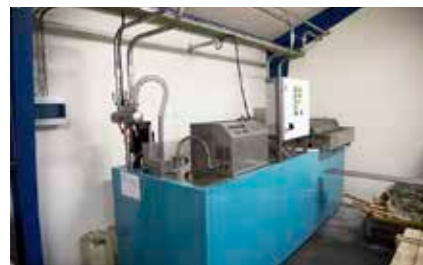
The central filtration system for filtering coolant.
