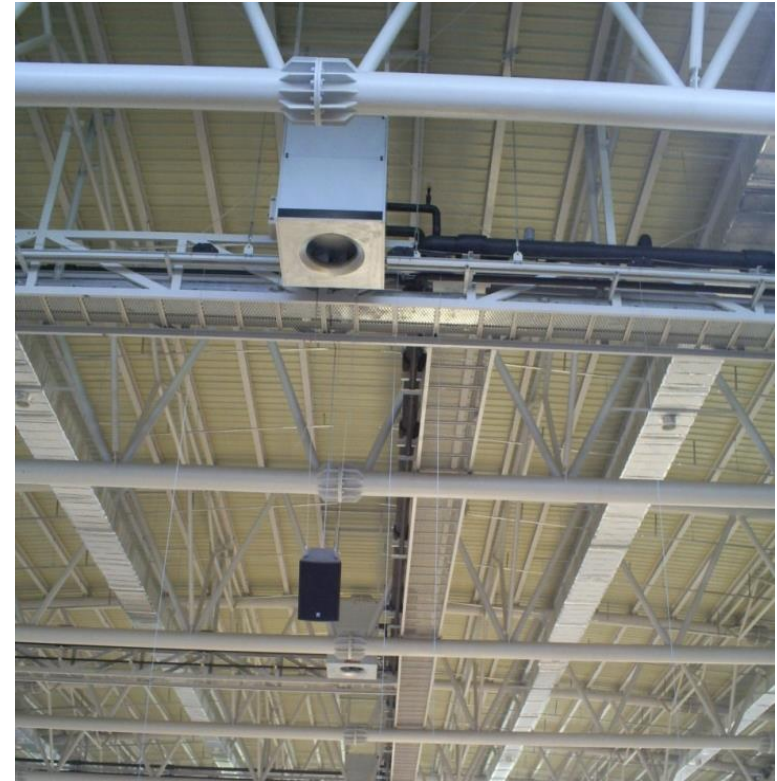
DCF-11 installed at Korea National University Tiger Dome, Seoul
