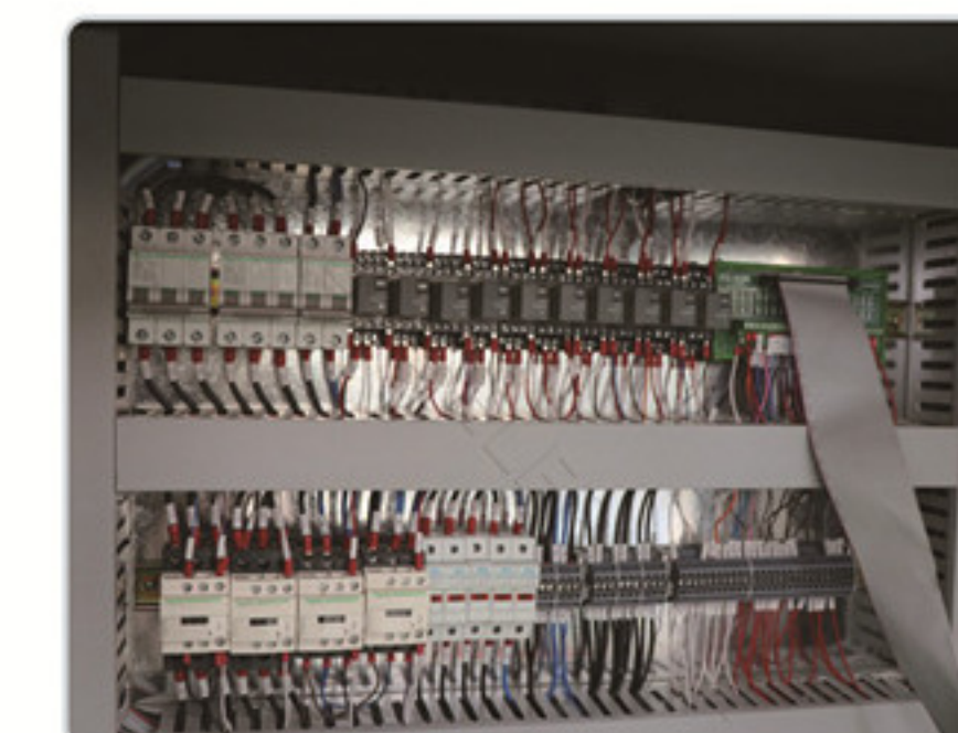
High quality Schneider electric
