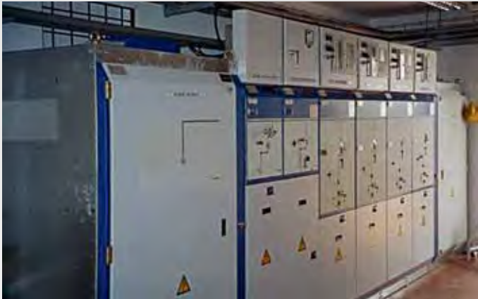
ABB Substation - MOZAMBIQUE - ORMAZABAL CGM 36kV, 8 fack
