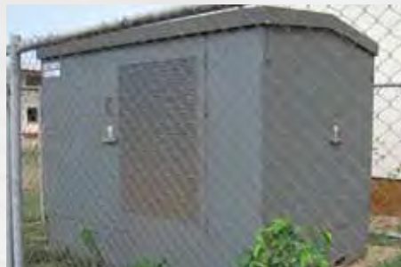
Military Housing Monrovia - LIBERIA - SEBAB utomhusstation 11kV
