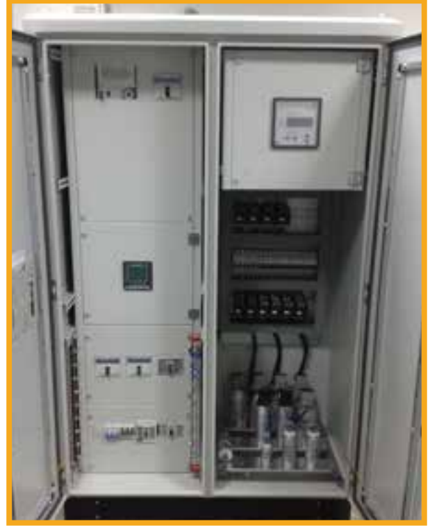
OUTDOOR CAPACITOR BANK APPLICATIONS
