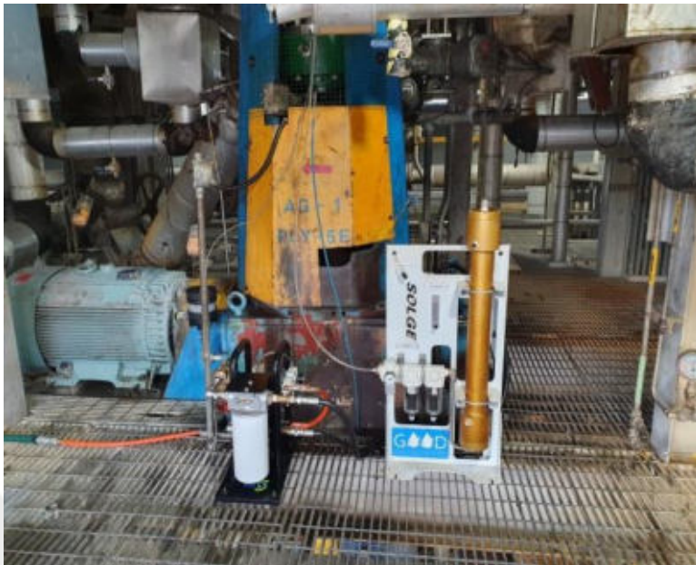
[EHC unit of Steam Turbine]
