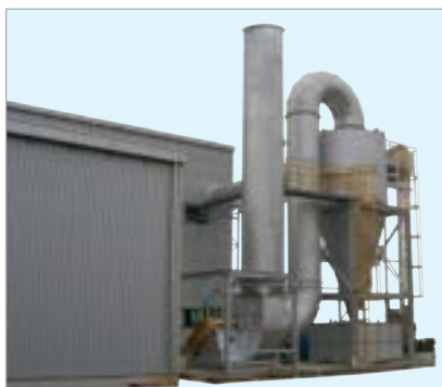
Venturi cyclone for nonferrous metal melting facility
