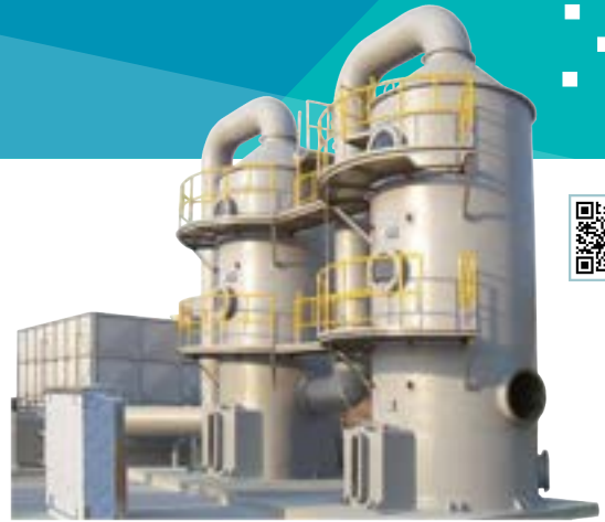
Odor Capturing at Sewage Treatment Plant
