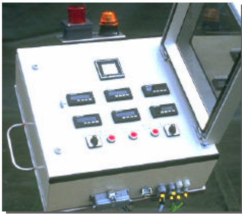
Fig.5. The local operator panel.
