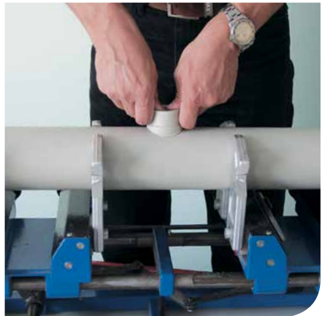
4. Put the heated saddle on the heated hole and fasten for about 16 seconds. You can fill the pipe with water and expose it to pressure one hour later.
